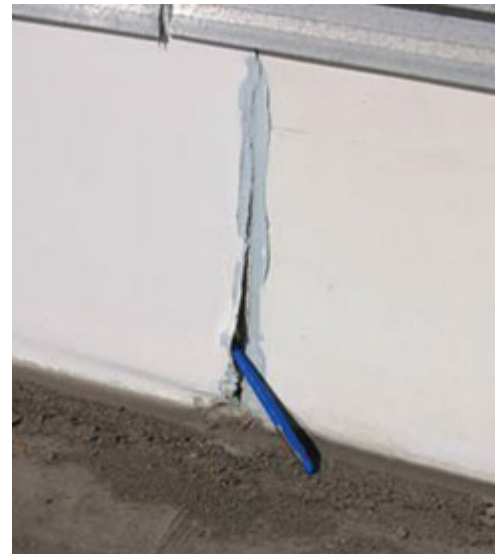
Photo 1: The soiling of this white membrane has resulted in a surface color darker than what would be experienced on a smooth-surfaced black roof covering.
