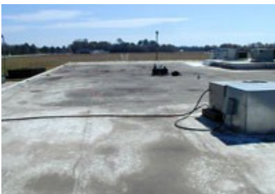
Photo 2: This photo shows the reality of a white roof surface membrane used in areas of heavy agricultural activity. The soil atop the membrane certainly has robbed the roof of its potential energy savings. Rather than trying to repeatedly clean the roof surface, using ballast would have been a better design choice in this situation.
