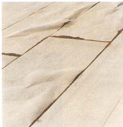
Figure 1: Blistering of a mop-applied SBS-modified bitumen sheet.
