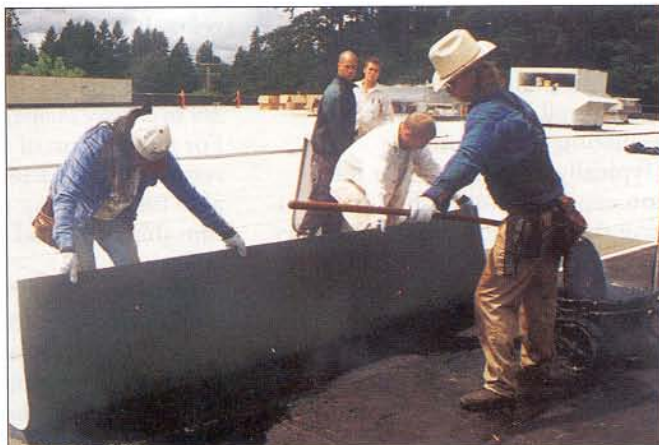
Photo 3: One worker prepares to finish mopping the roof area while two other workers flop a cap sheet.
