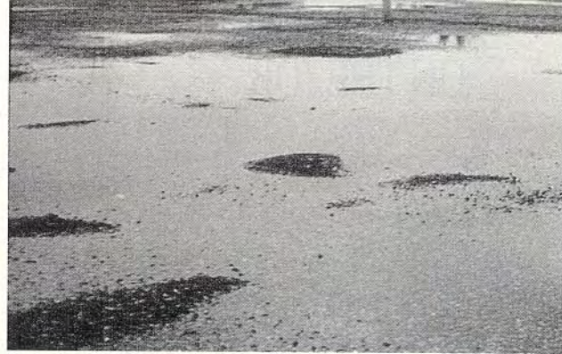
Even with design efforts to the contrary, ponding water is still a common occurrence in low-slope roofing.
